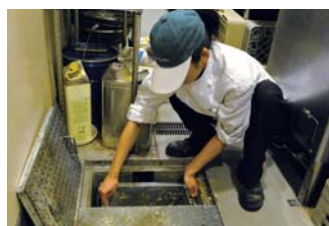
Grease trap cleaning
